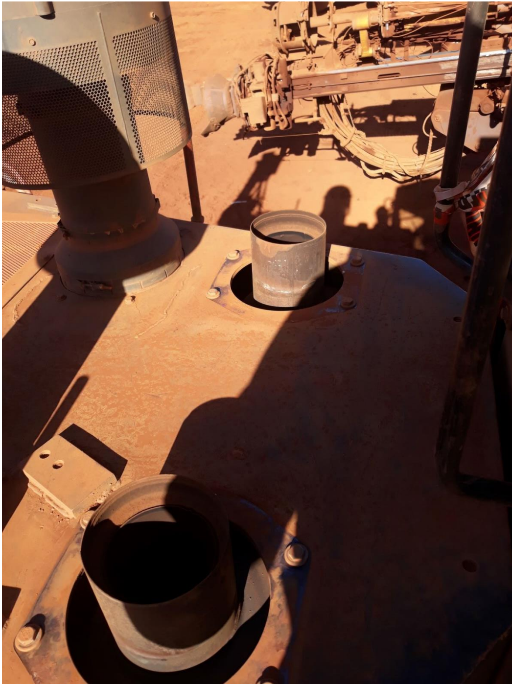
Top Engine cover with Exhaust stacks removed
