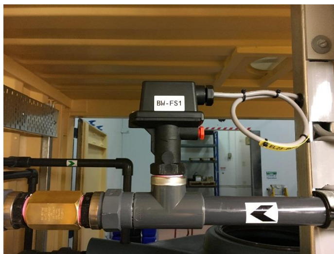
Backwash Flow Switch PP-FS1
