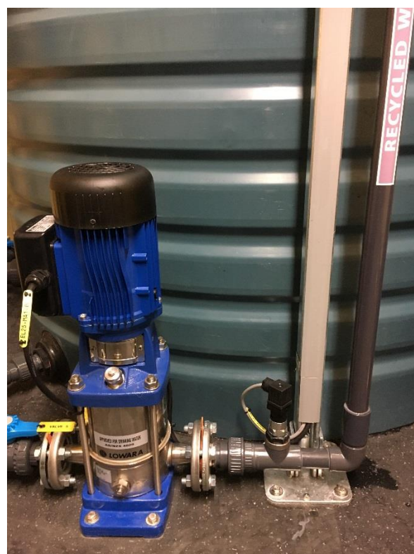
Polishing Pump Inlet Pressure Switch PP-PS1
