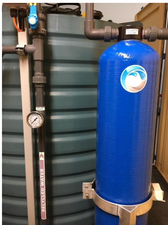
Polishing Filter Inlet Pressure Gauge
